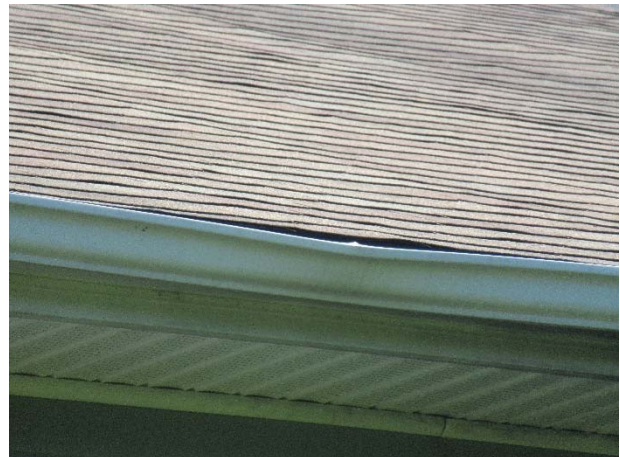
Gutter deflection (124 Sedum Road shown)
