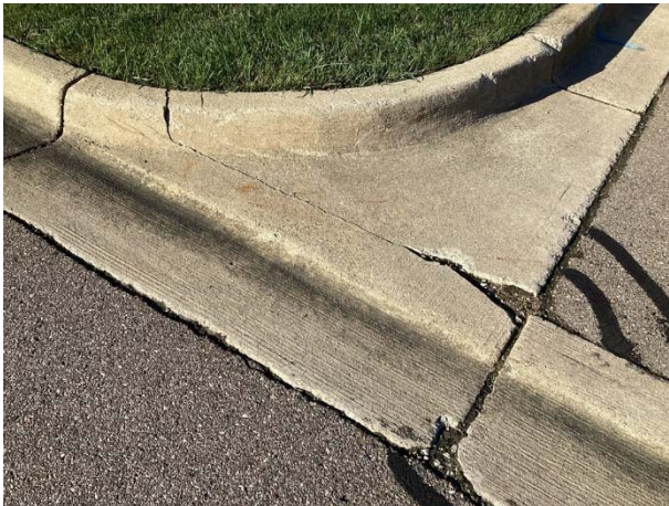
Curb and gutter cracks
