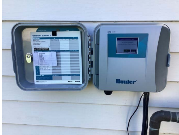
Irrigation system controller
