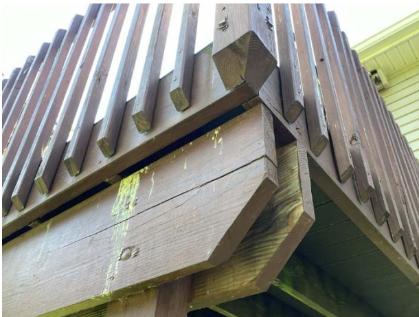
Beam crack (86 Sedum Road shown)
