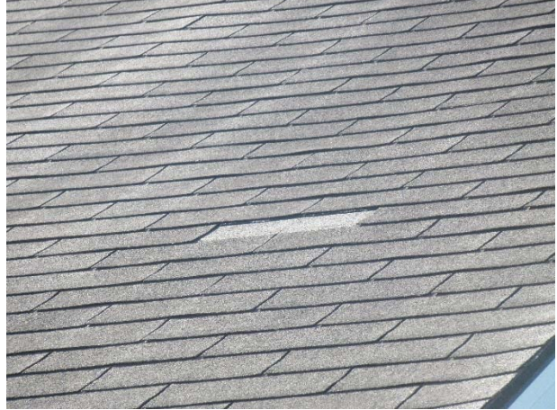
Missing shingles (160 Sedum Road shown)
