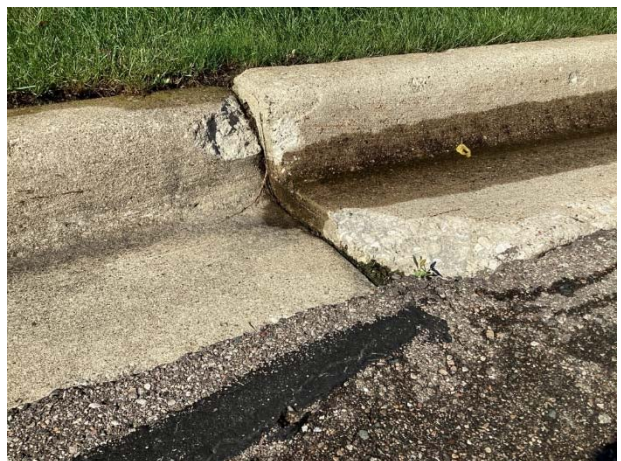
Curb and gutter settlement and spalls
