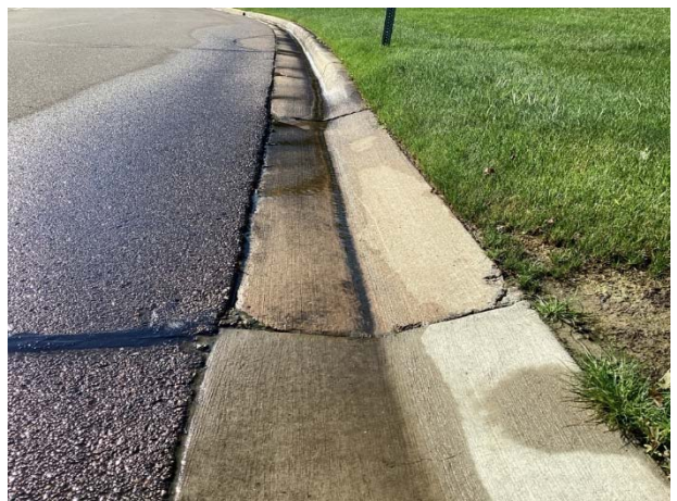
Curb and gutter settlement
