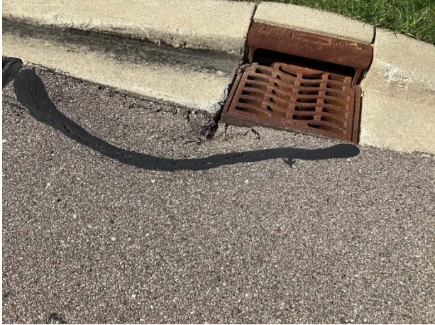
Pavement settlement at catch basin
