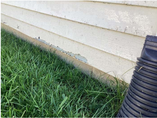
Siding damage (48 Sedum shown)
