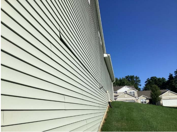
Loose siding (95 Sedum shown)
