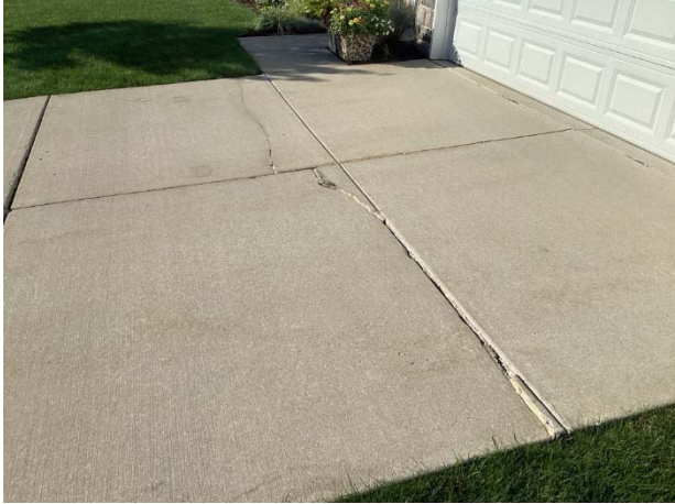
Driveway cracks (1038 Yarrow shown)
