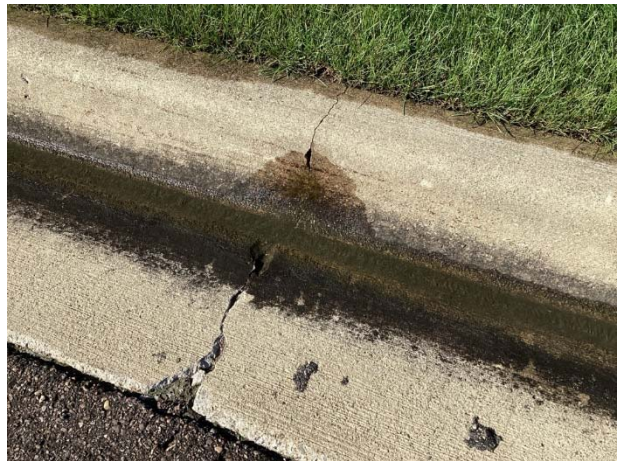
Curb and gutter cracks
