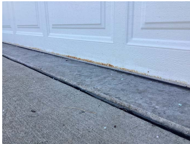
Base panel rust
