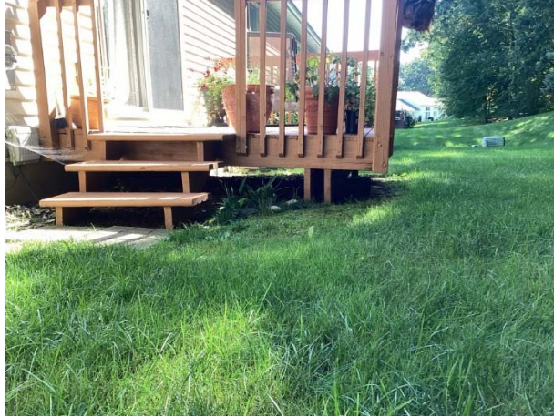
Deck settlement (886 Spirea shown)
