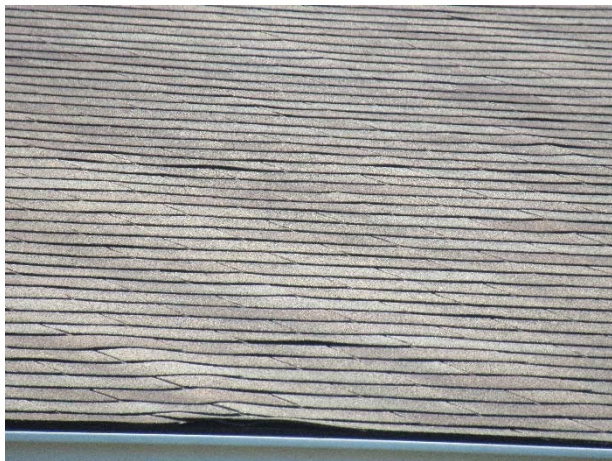
Sheathing deflection (112 Sedum Road shown)
