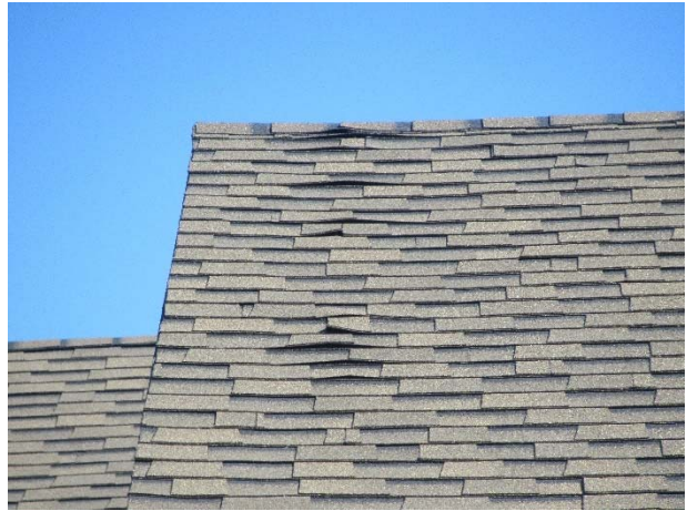
Nail pops (103 Sedum Road shown)
