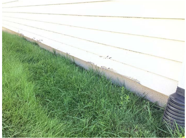
Siding damage (470 Hostra shown)
