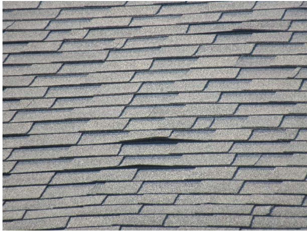
Nail pops (122 Sedum Road shown)
