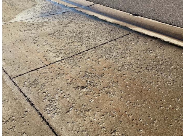
Sidewalk spalls and settlement at curb
