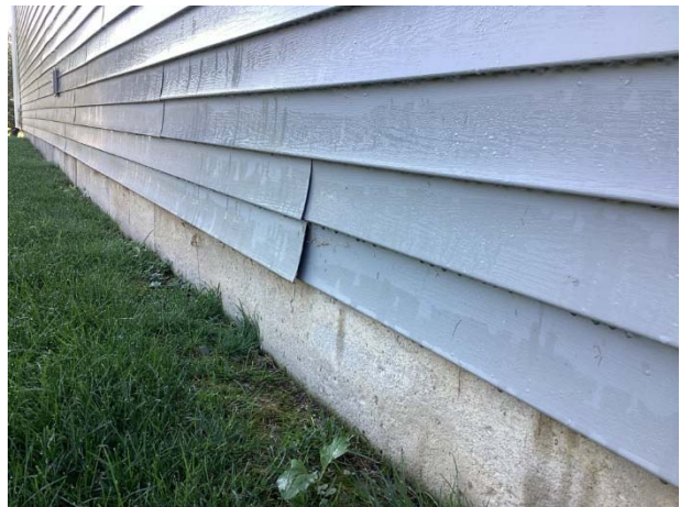
Loose siding (1038 Yarrow shown)
