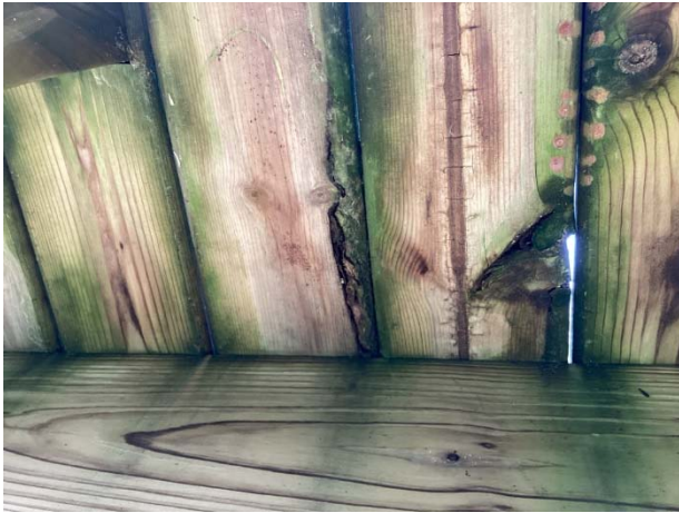
Deck board rot (99 Sedum Road shown)
