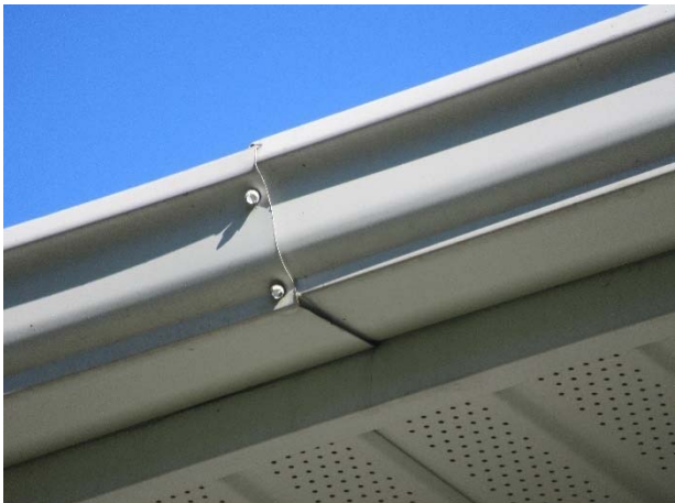
Gap in seam (99 Sedum Road shown)
