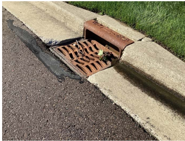
Catch basin settlement
