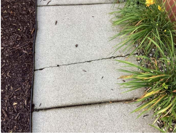
Sidewalk cracks (16 Sedum Road shown)
