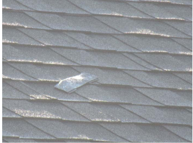
Loose shingles (1044 Yarrow shown)
