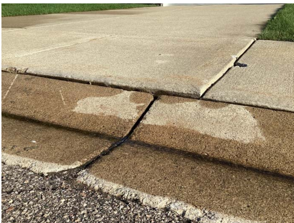
Sidewalk upheaval (152 Sedum Road shown)
